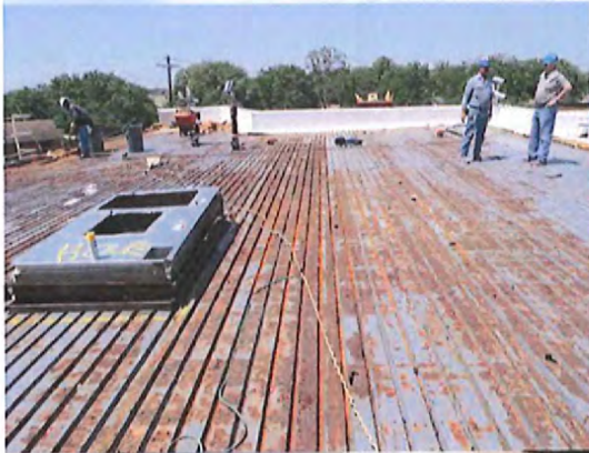
Rusted out decking
